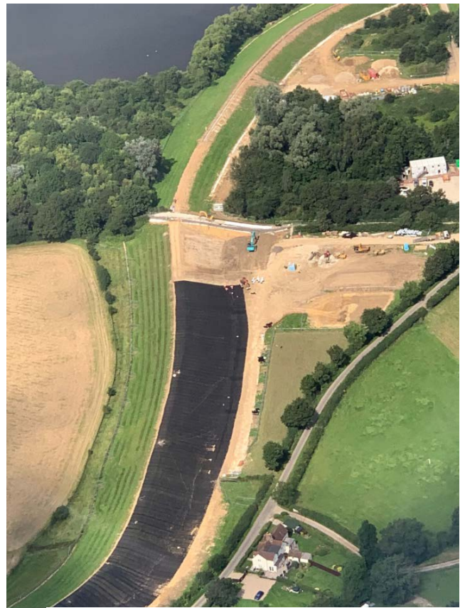
Reinforcing materials being laid on the main embankment of the Leigh FSA
